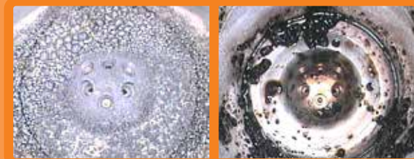
BEFORE: Injector with heavy deposit buildup
