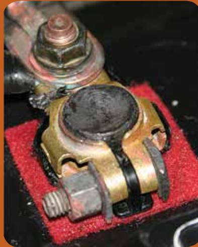
Battery terminal after BG Battery Service
