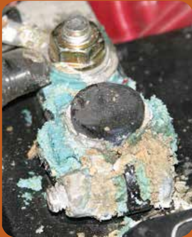
Battery terminal with corrosion buildup
